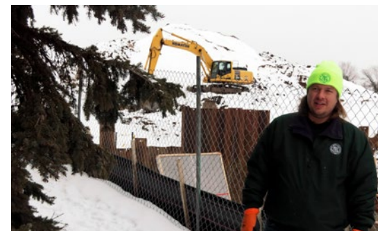
City Forester Luther Overholt stands inside the fencing that protects a fir tree and its critical root zone from pump station construction at West 72nd Street and Oaklawn Avenue. (Photo by Tom Cornell)
